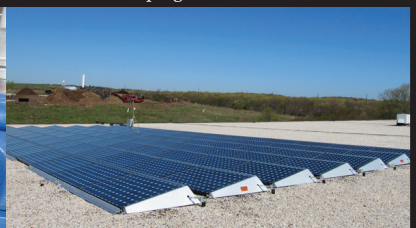
Smithtown Solar Photovoltaics
