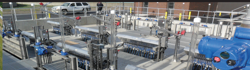
Bergen Point UV Disinfection
